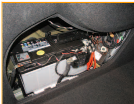
12V battery in luggage compartment with main fuse box
