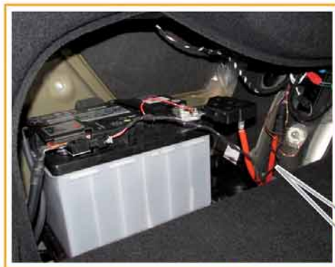
12-volt vehicle battery
