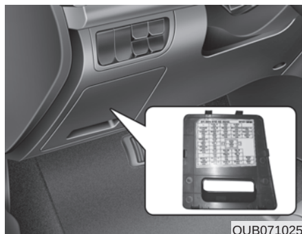
Instrument panel fuse panel
